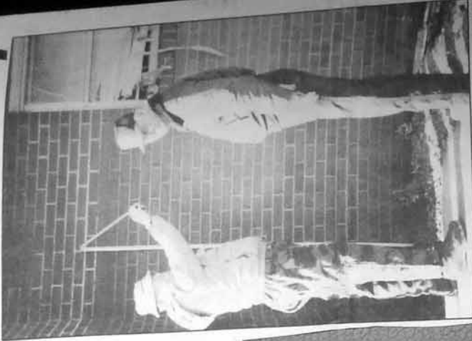
Ronceverte City Council member Tom Morgan and Chief of Police Bill Rose measure the high water mark on the front of Ronceverte's City Hall at 82 inches. All the front windows and doors were broken, and venetian blinds and assorted paper pokes through the broken window. (J. C. Browning photo)
